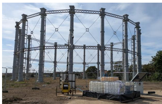
Figure A – Solar powered coal tar pumping system and bunded storage containers in operation at Hendon.
